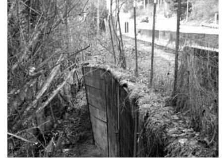
View of the challenged retaining wall with Oak Bay Road at upper right.
